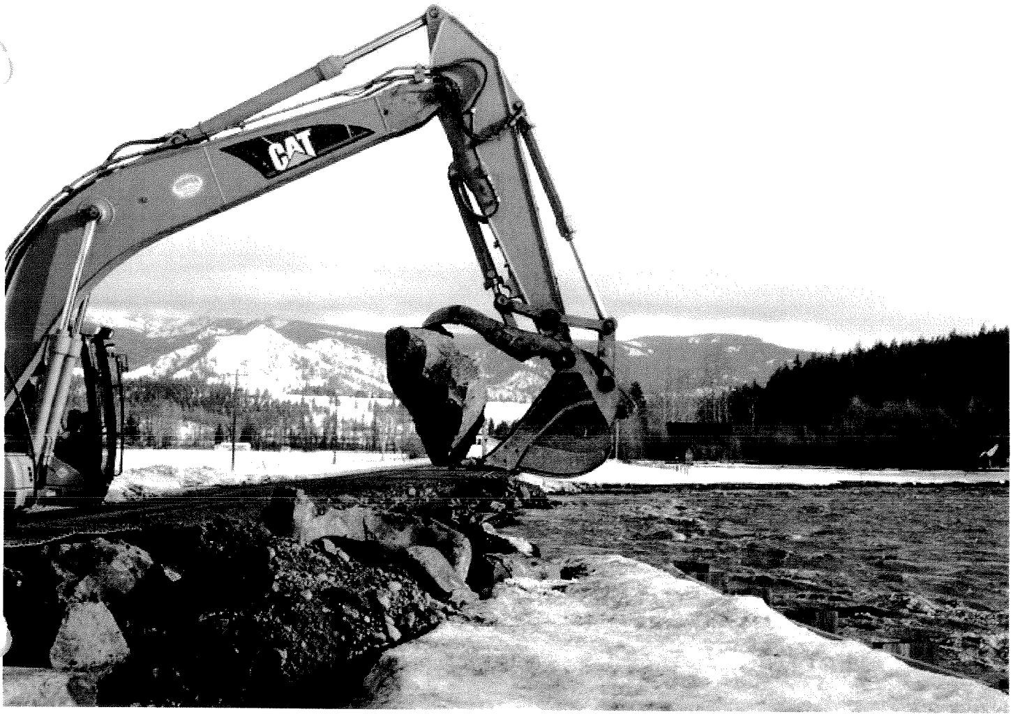
Where HWY 970 washed out.
